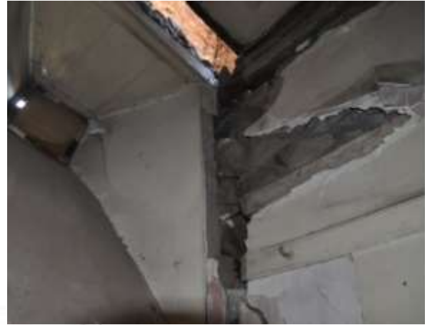
Fig. 8. Wide separation in the wall
